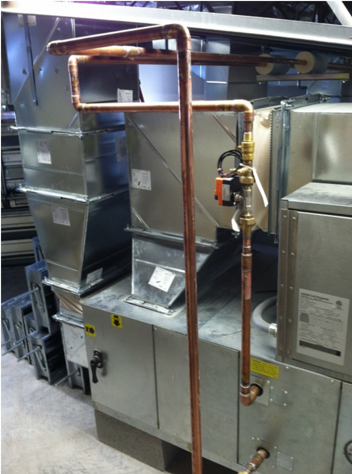
15-015 Supporting Image: Unstable piping
